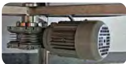
Close-Up of the Motor
